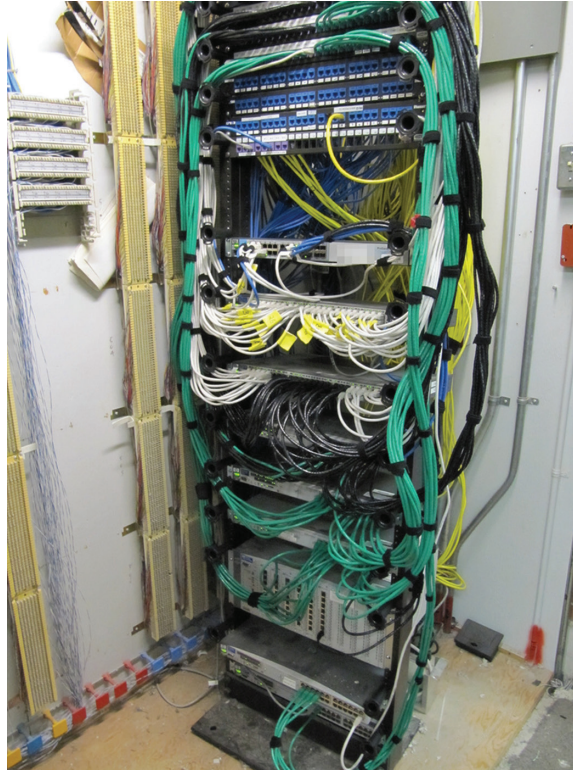
FIGURE 10.1 A typical wiring closet
